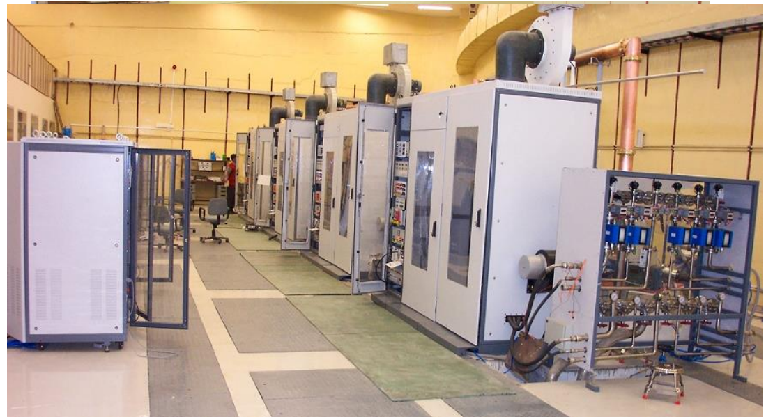
Indus-2 RF equipment Hall
