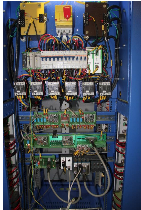
Electrical and embedded control sub systems
