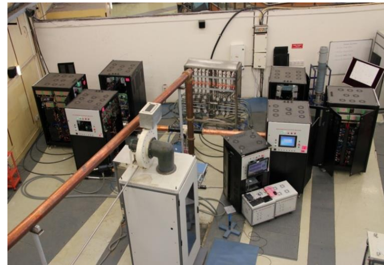
Fig 4: 75 kW SSPA coupled to RF cavity # 5
