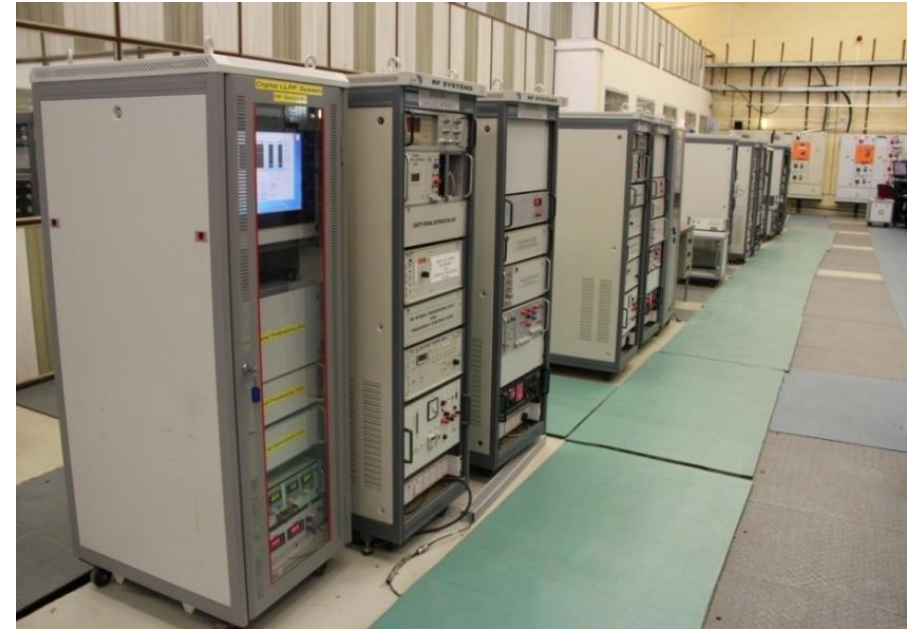
Digital LLRF systems installed in Indus-2
